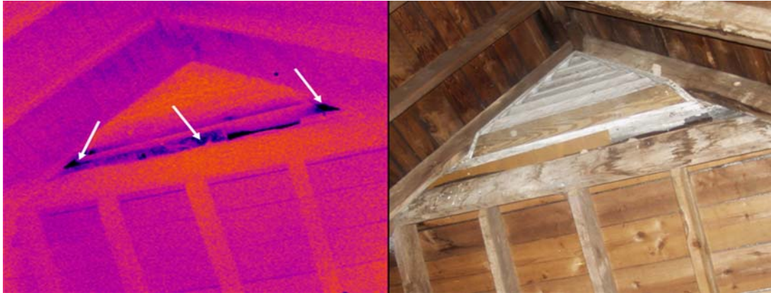
Figure 1 – Water entering the attic of a large church at the gable end vent.
