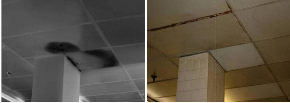
Figure 5 – Uninsulated column passing from cool area into the warm, moist interstitial space, causing condensation on the column, which then drips onto the ceiling tiles.
