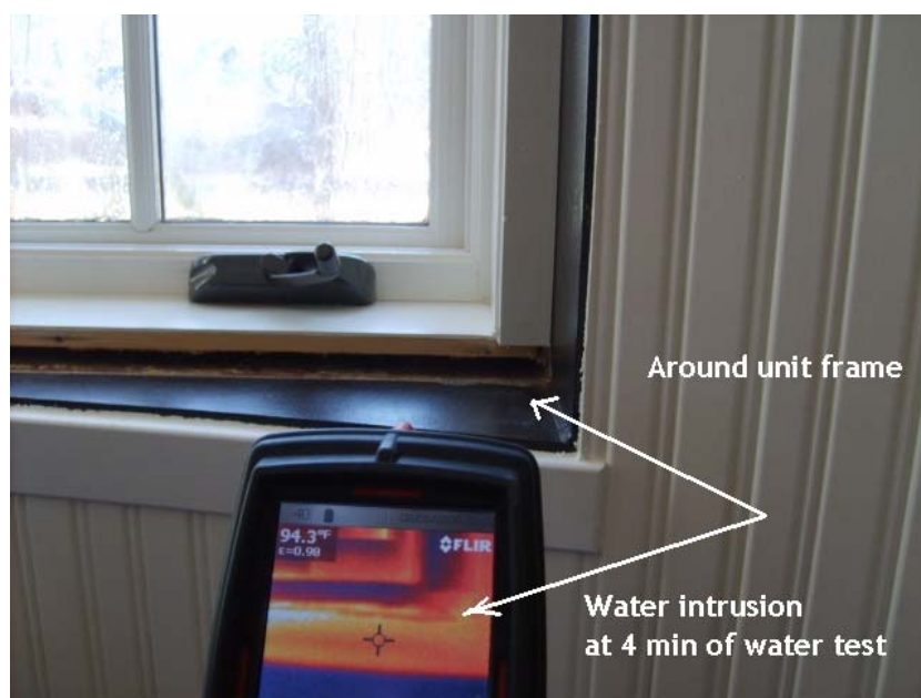
Figure 9 – Infrared imager documents water intrusion.
