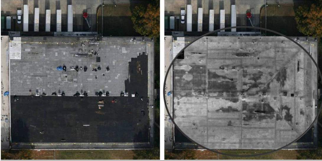
Figure 6 – Flat roof with wet insulation (lighter gray) being covered with new coatings.
