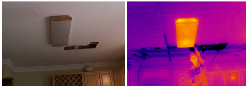
Figure 4 – Plumbing fixture leak in a house, found in seconds with an infrared imager.
