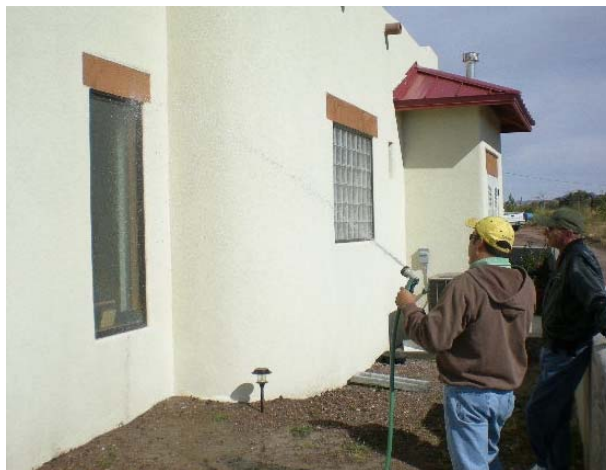
Figure 7 – Non-calibrated hose test being performed.
