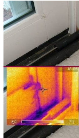
Figure 3b – Water intrusion at a door.
